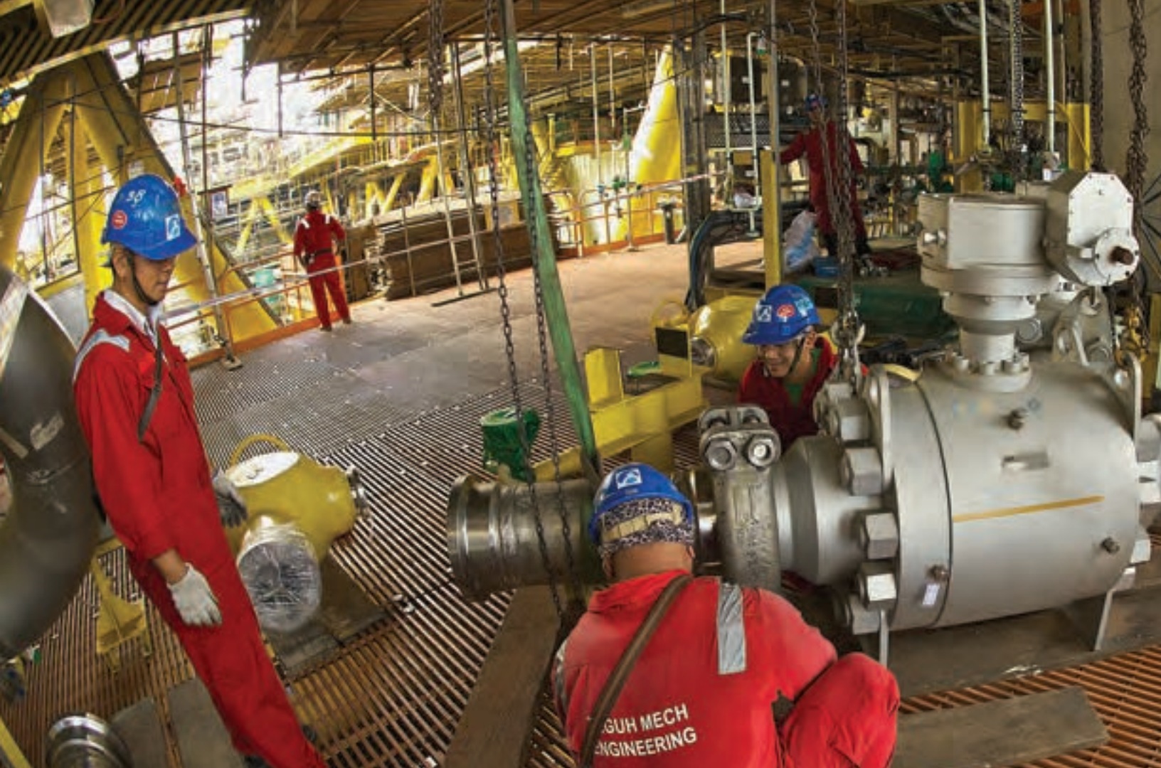
Above: Workers complete installation of heavy equipment before commissioning the Gumusut Kakap Platform.
